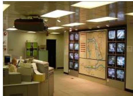
ATC Control Room
